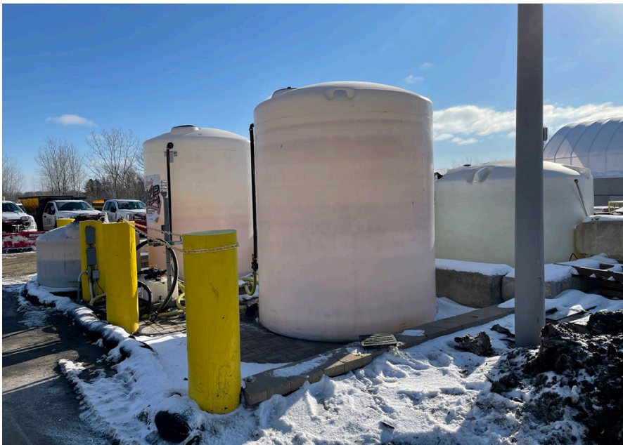
Plastic liquid storage tanks protected by concrete ballasts to prevent vehicles from hitting the tanks.
